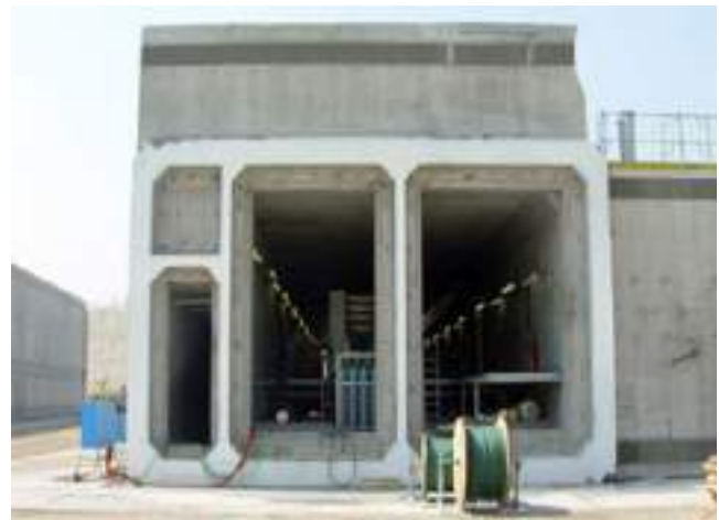
Concrete element with maintenance walkways and supply conduits
