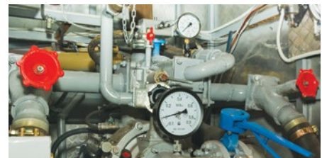
Pump and valve control
